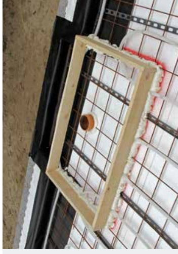
Before moulding the concrete deck, fit a wooden box (width 125 cm x depth 100 cm) into the insulation material
